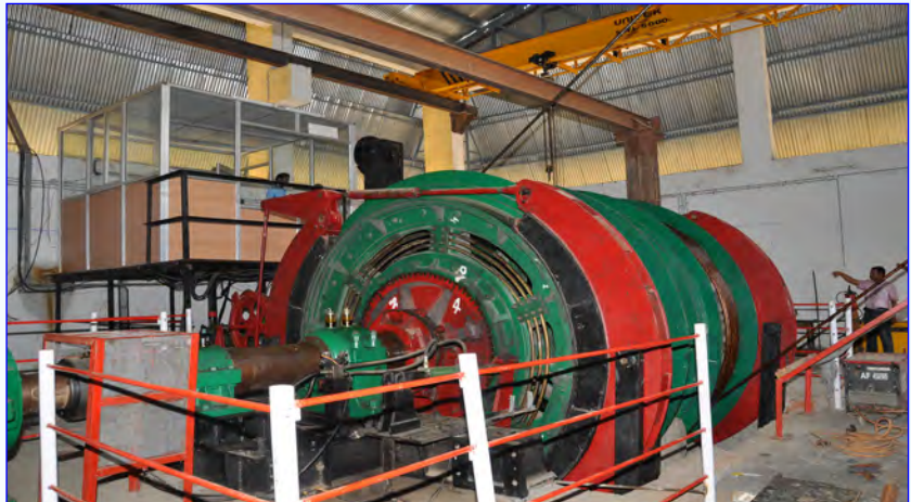
D.C. Winder installed at MOIL's Mine
